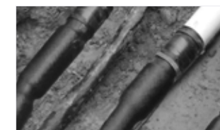
MV underground networks
