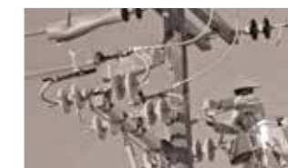
MV overhead networks
